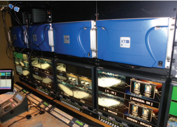
EVS servers. Depending upon configuration, each box can have up to eight IO channels, although boxes that handle 1080p or 3D can have only up to six. Sometimes they are mounted where they are visible, though often they are mounted out of the way, as there are no operator accessible features activated from the box.
